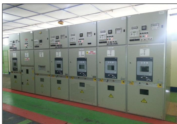
Figure 1. Physical example of external view 1: 20 kV medium voltage switchgear (Source: PLN)
